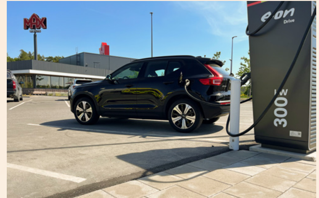
One of 254 electric car charging points at a MAX restaurant in Sweden.
